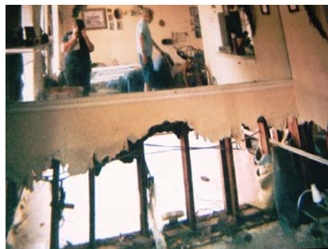
Over 3 feet of water flooded the Hart's home.
