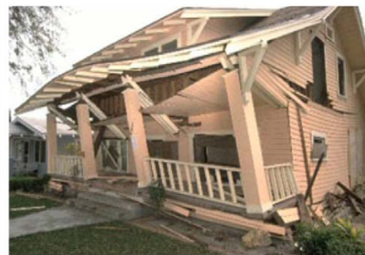
Volunteers and home owners have reduced earthquake damage in the Seattle region by retrofitting homes. – Seattle.gov/emergency
