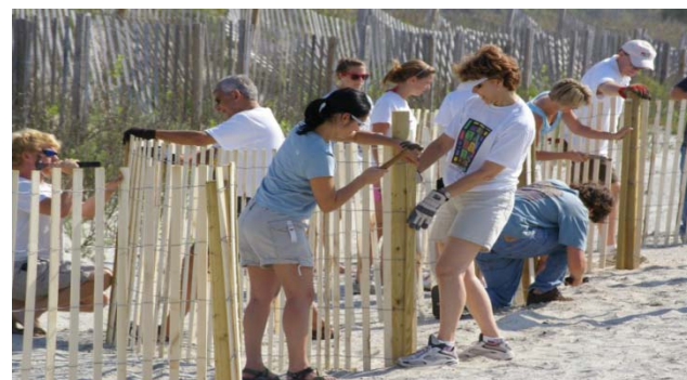
Volunteers install fencing to capture sand and create protective dunes on Folly Beach, SC. -Charleston Project Impact
